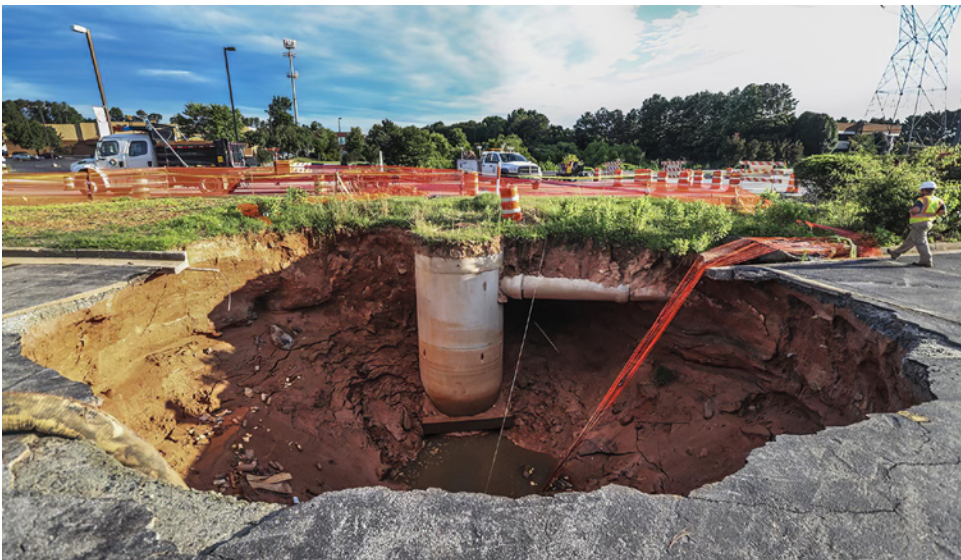
Sinkhole caused by leaking drainage pipe, Gwinnet, County, GA, June 2018 ( ajc.com/news/photos-few-metro-atlanta-biggest-sinkholes )
